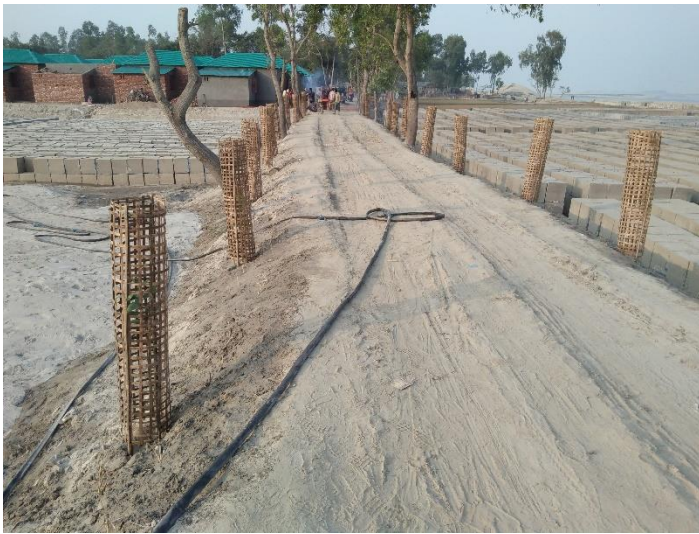
2 KM road renovation from house of Achars of Tetulkandi village under ward No 2 to house of Robiul of Mojartari village at Ranigonj,Chilmari
